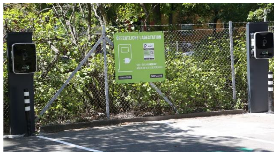
Berlin, EV Charging Infrastructure
